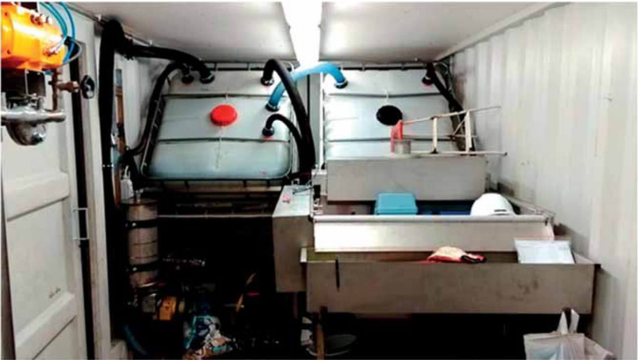
Picture 2: EGR wash water tank and purified water tank
